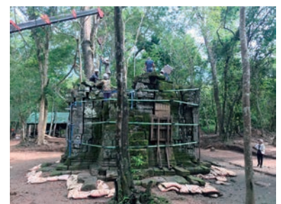
Restoration work of the east gate of Ta Nei Temple site in Angkor, Cambodia
