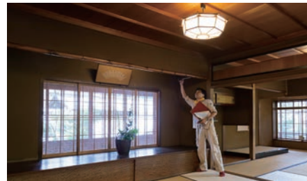
A building investigation on Ryotei Susaki in Takayama City (Nara National Research Institute for Cultural Properties)
