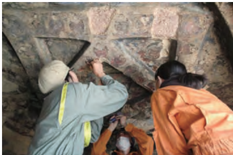
N(a)窟の保存修復の様子 (バミヤーン遺跡、アフガニスタン) Conservation intervention at Cave N(a) (Bamiyan Site, Afghanistan)
