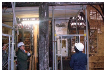
焼損した江袋教会の調査 Investigation of Ebukuro Church which was damaged by fire
