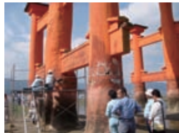
修復のための厳島神社大鳥居の調査 Examination of the torii of Itsukushima shrine for restoration
